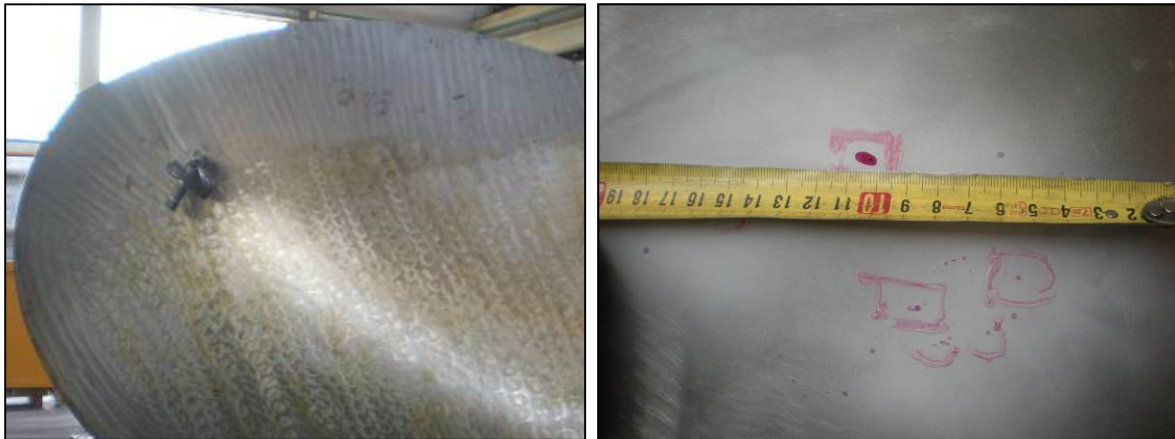
Fig. 3. Kaplan turbine blade: Defects on casting detected by means of Liquid Penetrant examination
