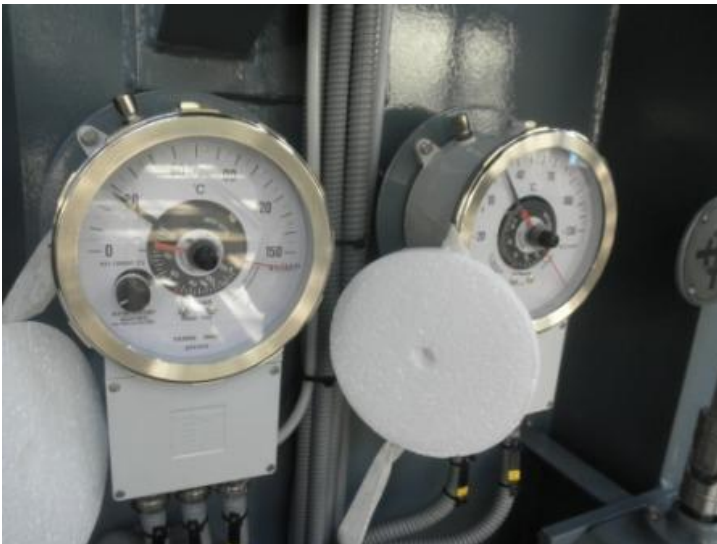
Details of the transformer
