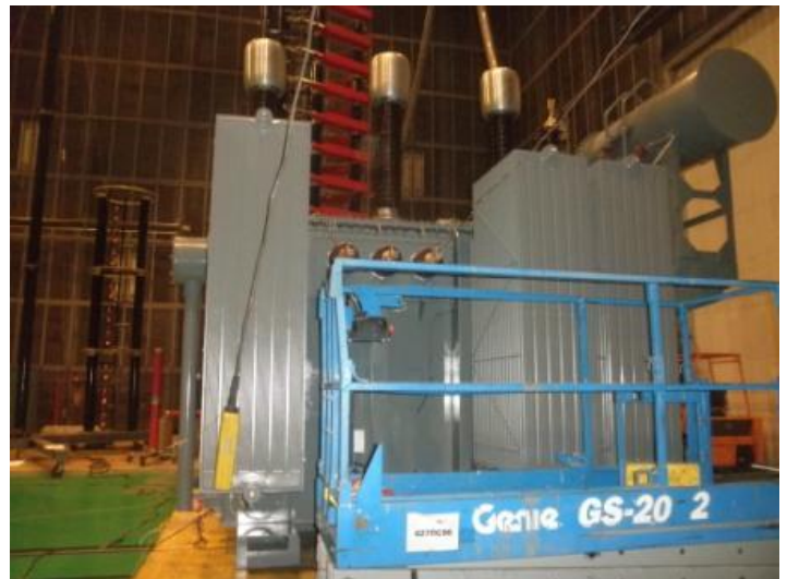
Transformer during the FAT tests
