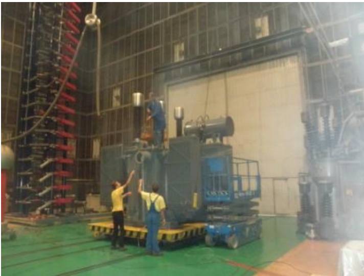
Transformer during the FAT tests
