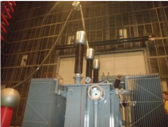
Transformer during the FAT tests
