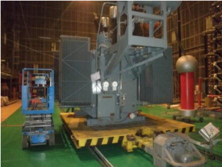
Transformer during the FAT tests
