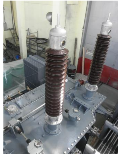
Details of the transformer
