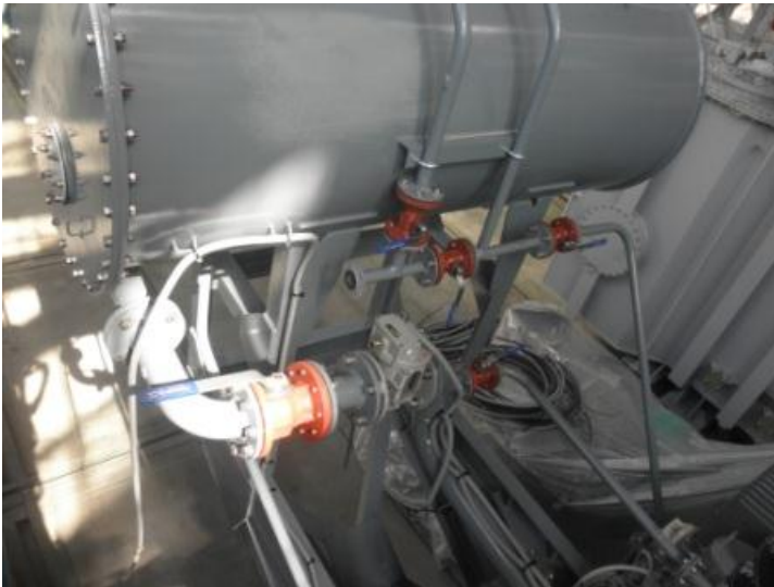
Details of the transformer
