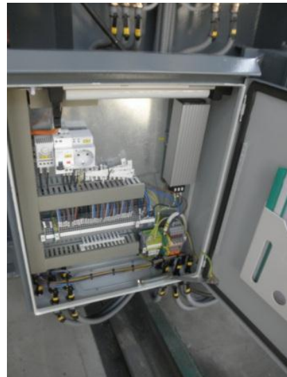
Details of the transformer
